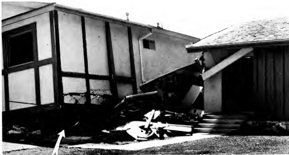
Photo 1. New split-level dwelling in the housing development southeast of Olive View Hospital. Garage under two-story level has collapsed (note crushed car).
